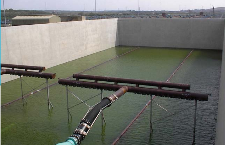
Floating solids excluding decanter
