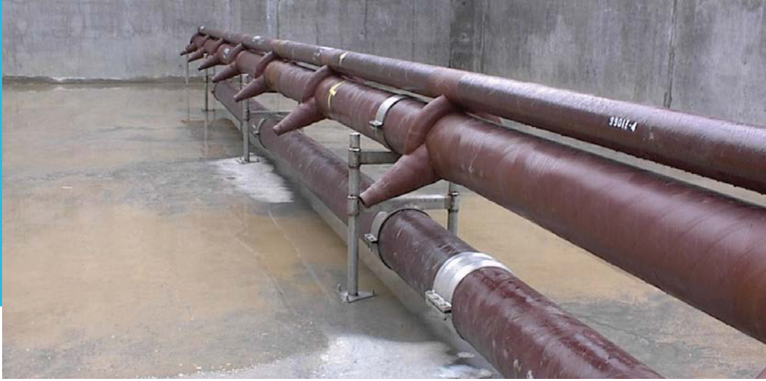
Influent distribution manifold
