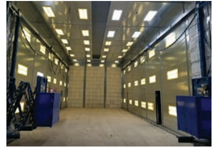
Climate Controlled Paint Booth
