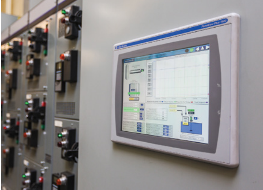
EFFLUENT TURBIDITY READING FOR SECONDARY CLARIFIER USING THE BIOMAG SYSTEM AT STURBRIDGE, MA
