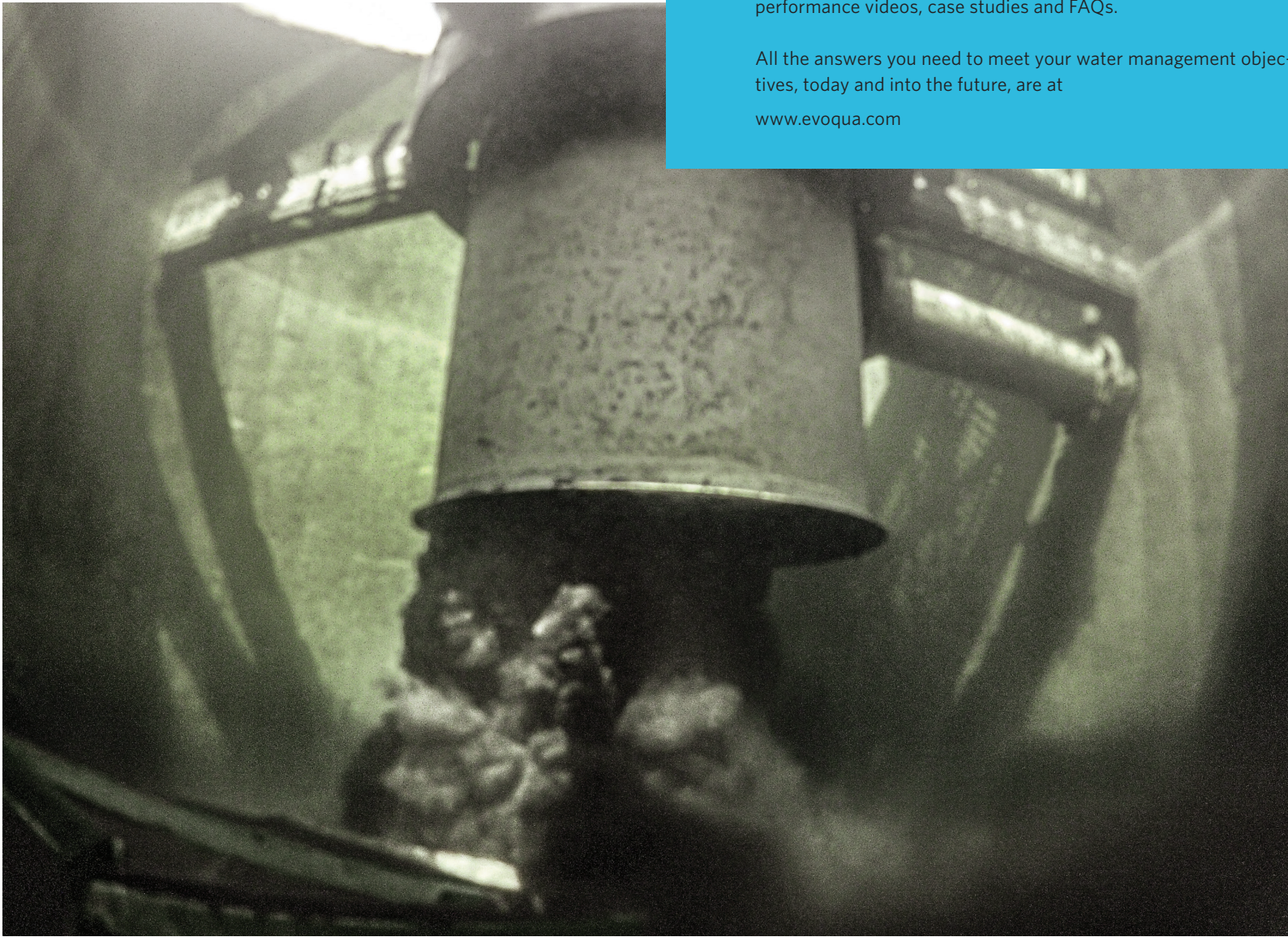
INSIDE A TERTIARY CLARIFIER AT STURBRIDGE, MA WASTEWATER FACILITY DEPICTING MAGNETITE BALLASTED TECHNOLOGY AT WORK
