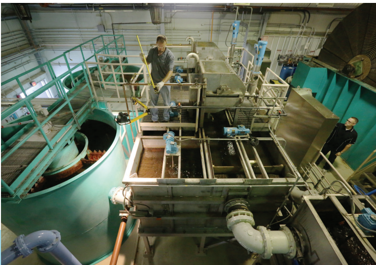
CHARLTON, MA. WASTEWATER FACILITY
