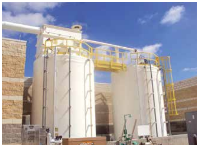
RJ-2000® Bulk Scrubber, Cypress WTP, Wichita Falls, TX
